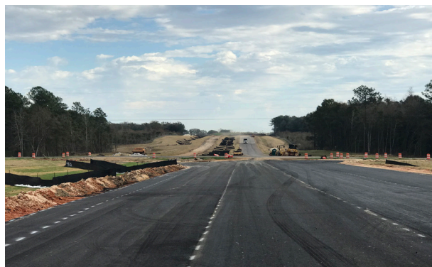
Initial asphalt layers on SR-158 extension from east of Glenwood Rd. to west of Lott Rd.
