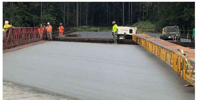
Deck pour for all four spans of the bridge over Seabury Creek. The bridge is now complete.
