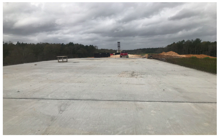
Crews have completed the deck pour for the bridge over Rogers Rd.
